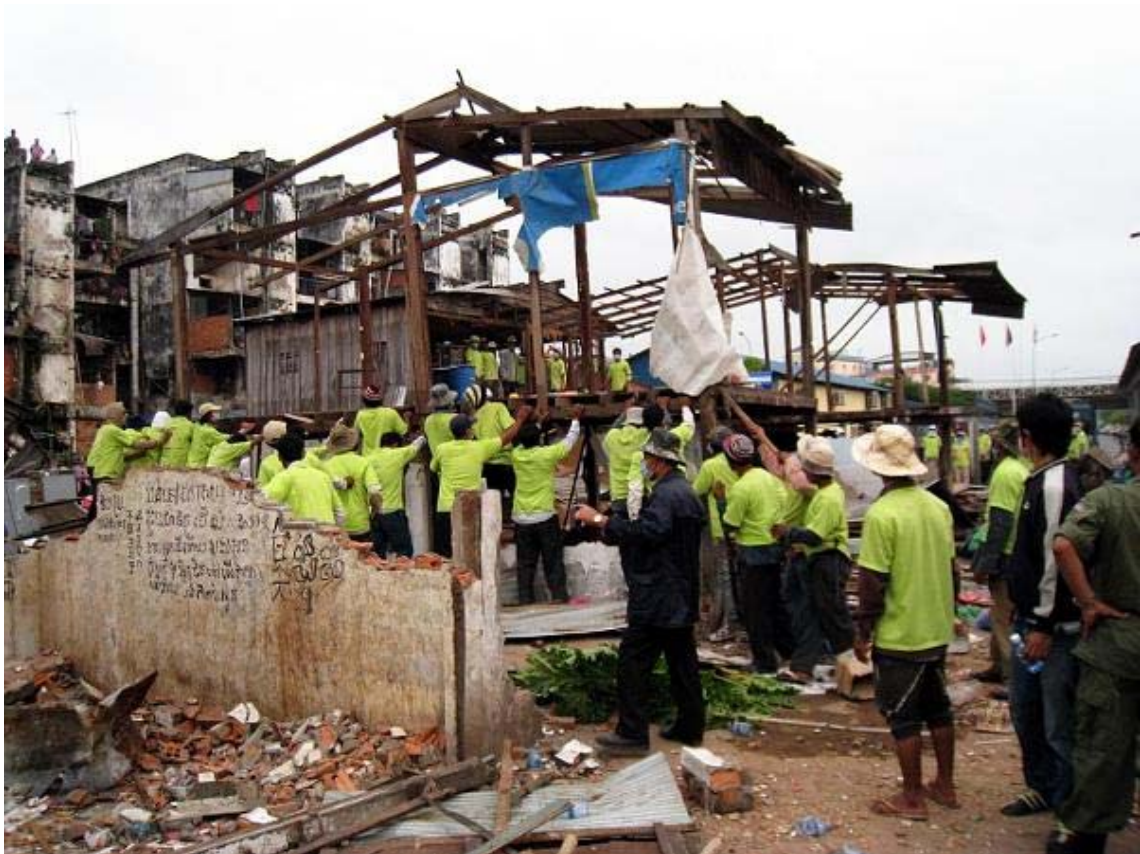
A line of workers push at the skeleton of a destroyed house, trying to topple it over.
